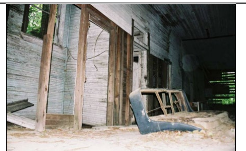
Page 227: Sims School: looking from fallen west side wall into west classroom; note loss of wall at west cloakroom and loss of beaded-board siding beyond.
