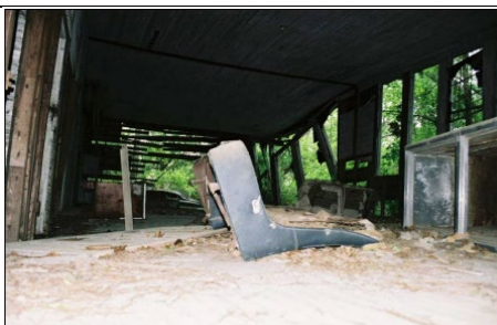
Page 227: Sims School: looking from fallen west side wall into west classroom and, at rear, east classroom; note absence of partition wall and damage to exterior walls.
